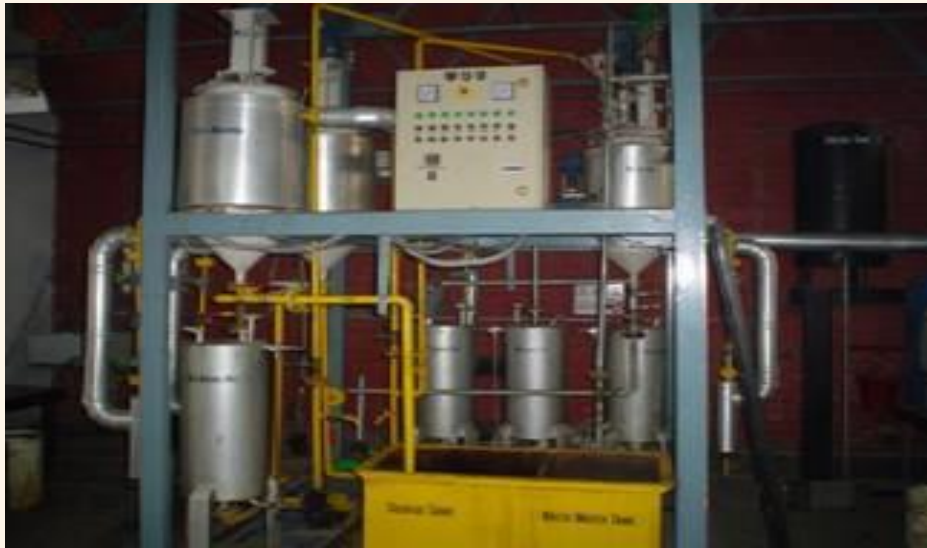
Figure 2: Biodiesel Pilot Plant
