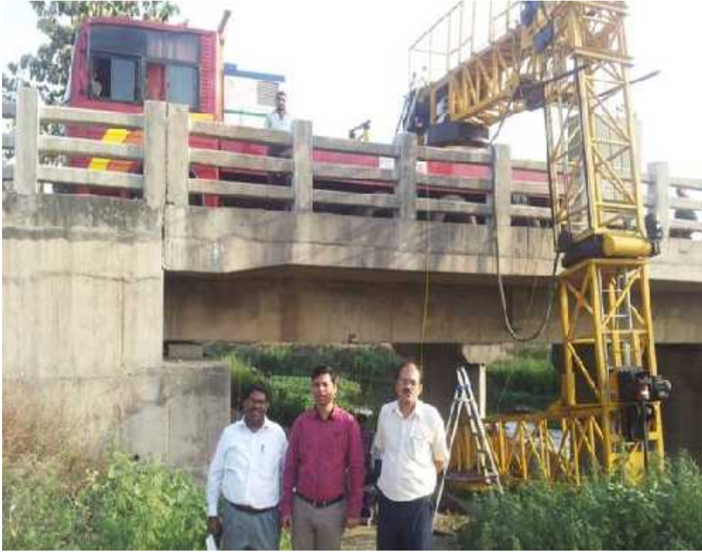
The MBIU under operation on a bridge enroute NH24
