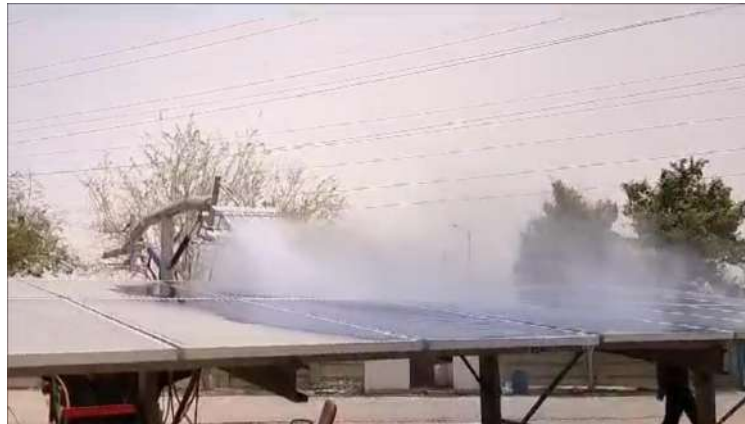
Figure: Demonstration of Dust Cleaning System at NTPC Bhadla
