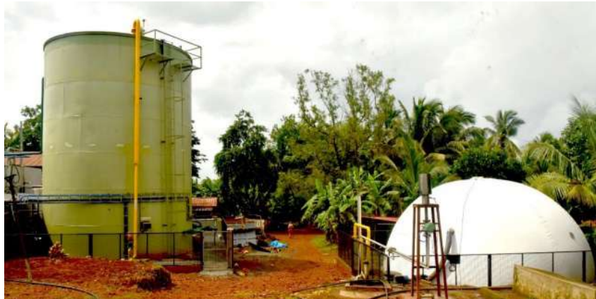
Figure: Sustainable bioenergy-based model effluent treatment plant for desiccated coconut industries at M/s. Vittal Agro Industries, Kasargod
