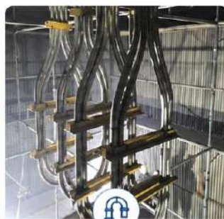
Test Loop at NTPC Dadri
