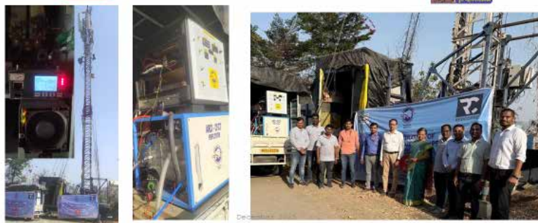
Fig. Airtel's Telecom tower with a maximum peak power operation of 4.8 kW was supported by ARCI developed PEMFC
