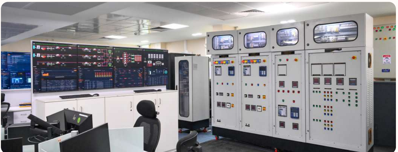
OT SOC & SCADA with PHIL (Power Hardware-in-the-Loop) Test Bed
