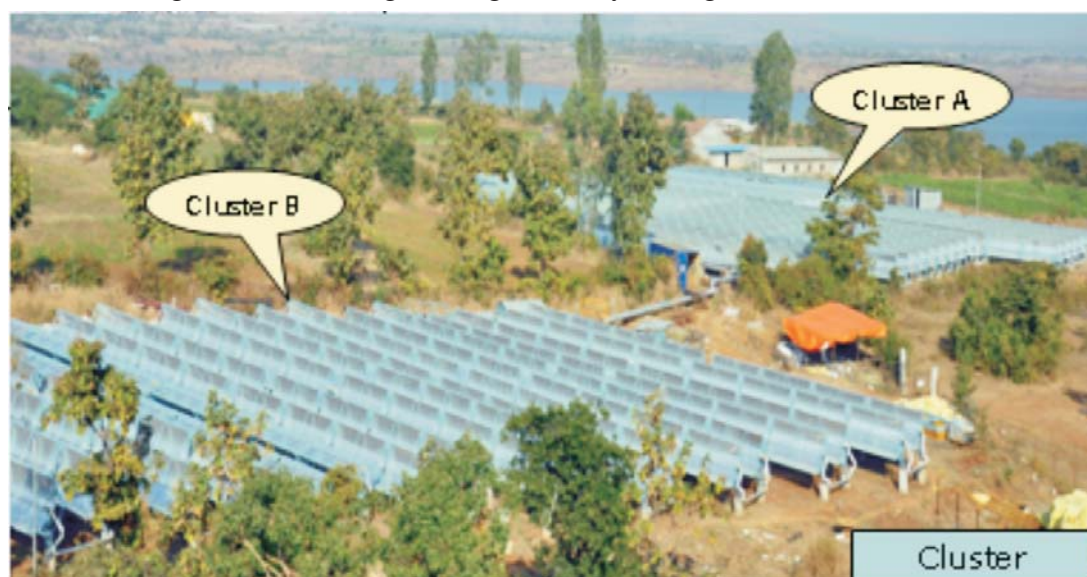
Fig. 4.32: Solar Field at Shive
