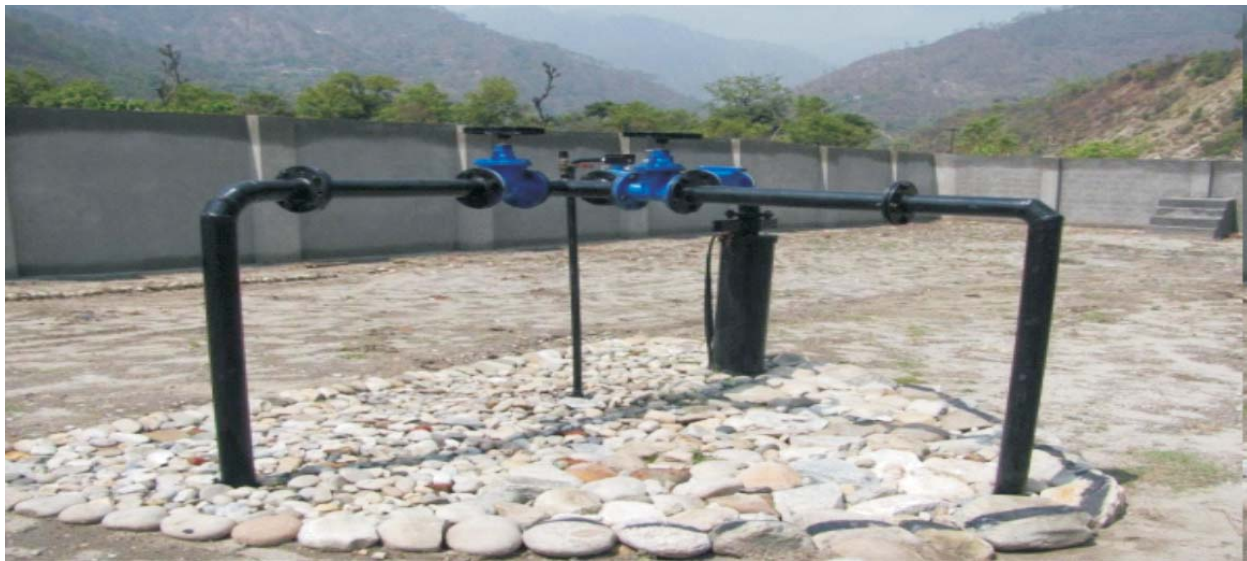
Fig. 4.36: River Bank Filtration well at Karanparyag
