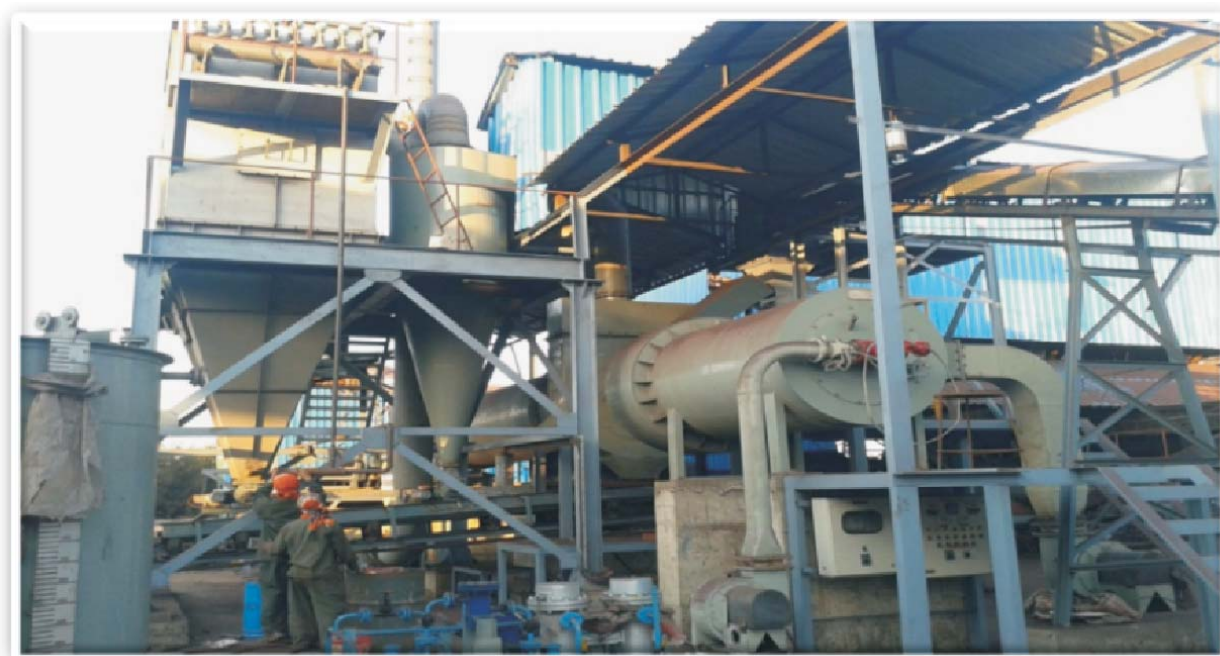
Fig. 4.73: Cyclone and Bag house
