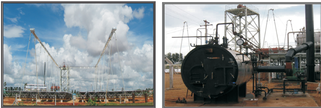
Fig. 4.33: Solar – Biomass Hybrid Sea water desalination plant in Ramanathapuram district of Tamil Nadu
